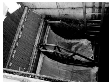
In 1999, North Bergen Municipal Utilities installed numerous mechanical screen bars and netting systems to control solids and floatables in CSOs. The facilities cost $3.3 million and annually cost $57,373 to operate and maintain (2002 dollars).
