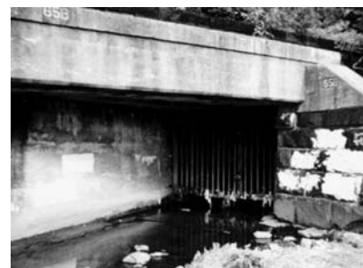
CSO outfalls were constructed in a wide variety of shapes and sizes, including the large box culvert shown here. In general, CSO outfalls discharge directly to receiving waters.
