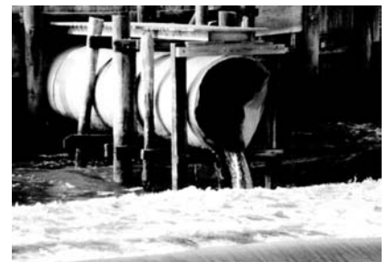
Typical CSO outfall discharge following a storm.
